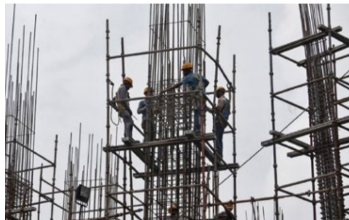
Workers erect scaffolding at a construction site of a metro rail station in Kolkata, India
